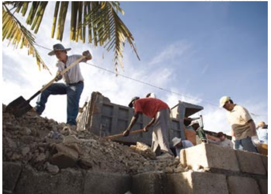
Herbert Funk, left, and fellow members of a Work and Learn Team from Paraguay clear away the rubble of Adral and Marie Sylvain's house in Port-au-Prince, which collapsed during the Jan. 12, 2010, earthquake. Clearing the property made it possible for the Sylvains, who work with MCC and have four children, to build a wood and tin-roof home.
