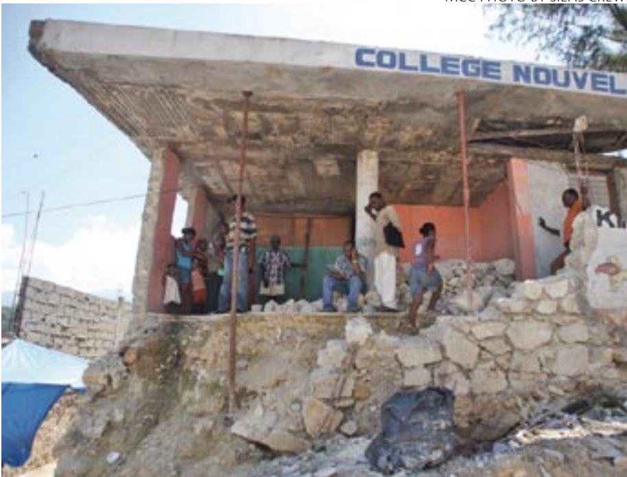
Structural engineer James Mwangi, a Mennonite Central Committee worker, seated, and a team of Haitian engineers and masons pause while inspecting a building used both as a home and a school that was later repaired. The building is part of a project that includes home repair for 200 people living with disabilities.
