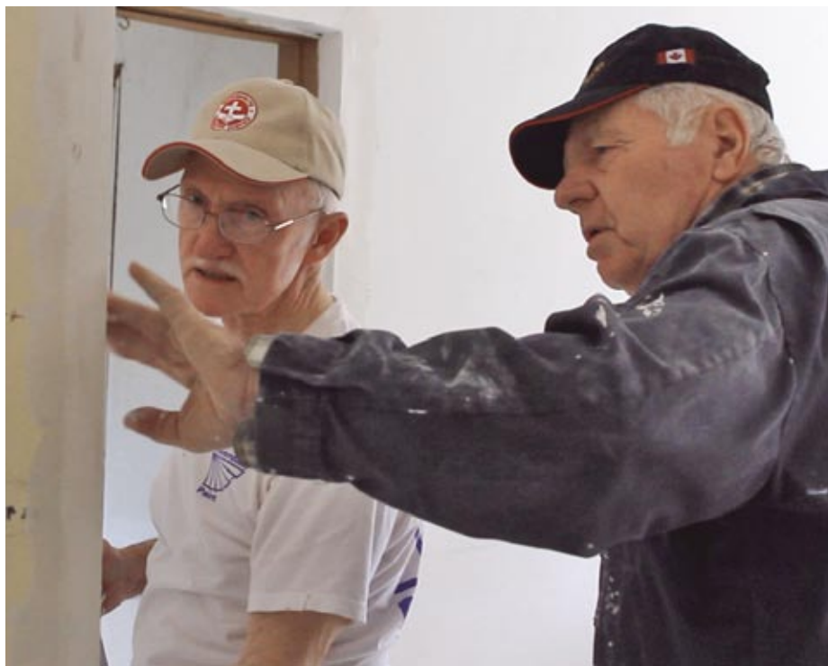
MDS volunteers Dave Friesen and Eric Penner examine the drywall finishing work they are completing.
