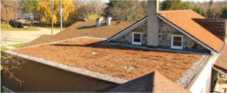
Last fall, workers installed a 'green' roof over the Stonehouse meeting room at Hidden Acres Mennonite Camp.
