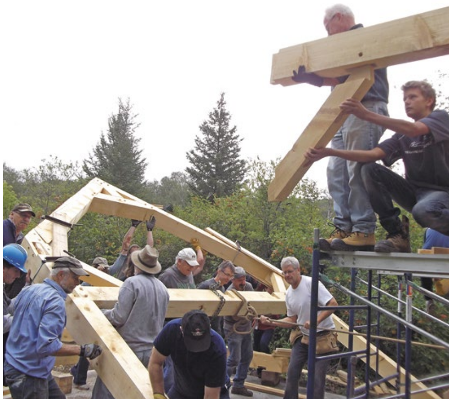
Volunteers raise the timbers of the second timber-frame cabin to be built this year at Shekinah Retreat Centre.
