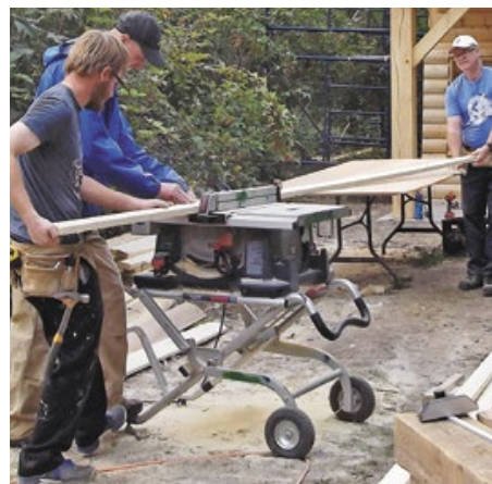
From left to right, volunteers Ryan Siemens, Curtis Wiens and Gord Siemens cut a board to be used in the timber-frame cabin constructed during the MDS Family Project held at Shekinah in August.
